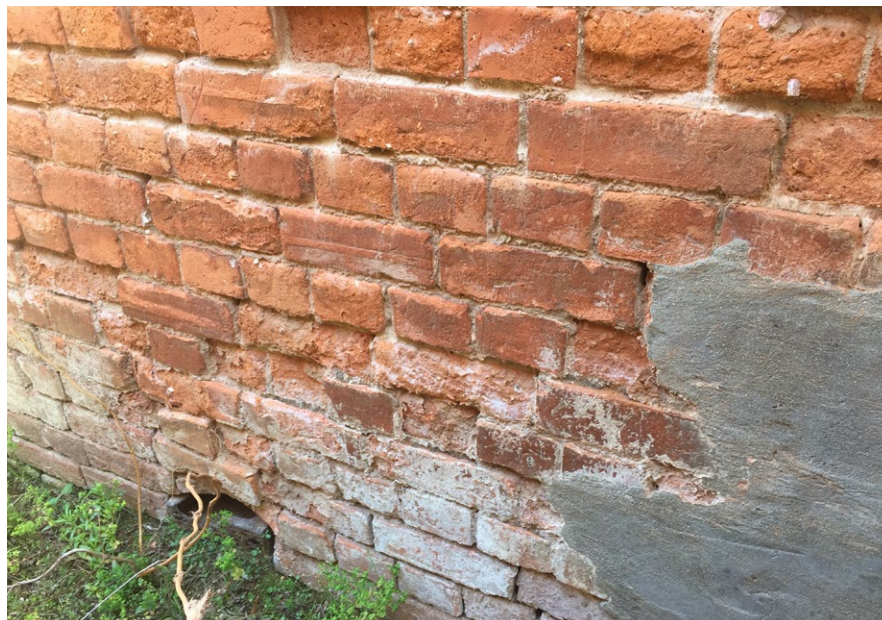
Drainage issues at the base of the building will result in movement in the shallow stone footings and consequent cracking of the walls.
