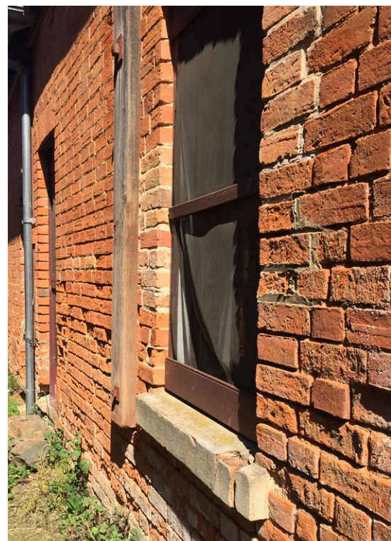
Rising damp and humidity carry more salts up into the brickwork. Salts on the wall surfaces will result in more rapid decay of the soft, porous brickwork.
