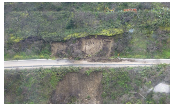
Landslips blocking and undermining the road. (Image: Department of Transport)
