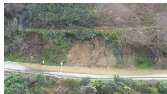
Flood damage along the road. (Image: Department of Transport)
