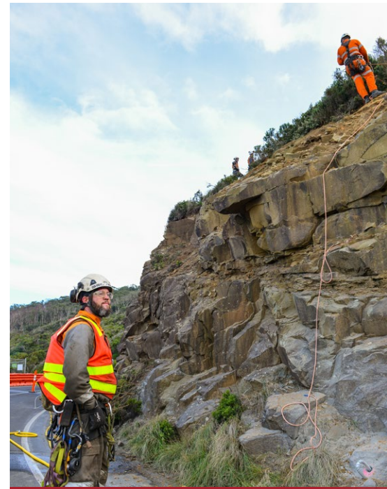
Work to prevent rockfalls and erosion beside the road. (Image: Department of Transport)
