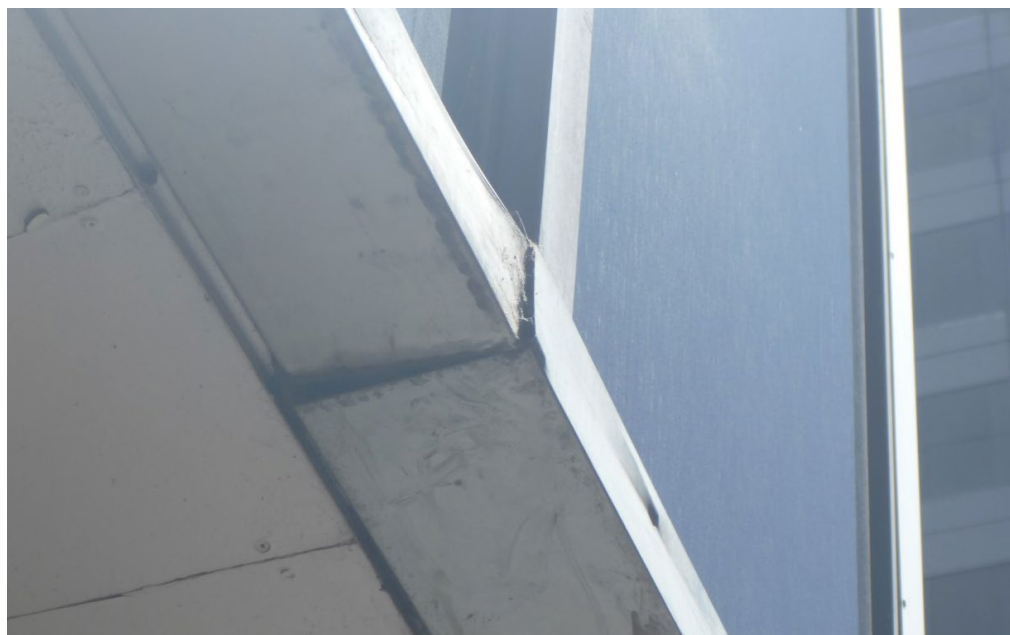
Climate change will accelerate deterioration of materials, e.g., more frequent and intense storms will lead to recurring damage to gutters.
