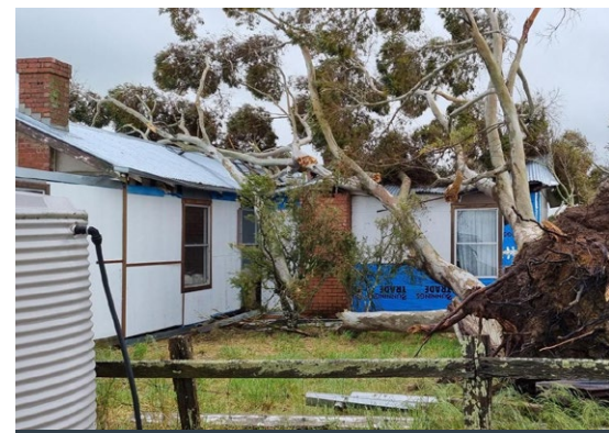
Roof damage to an outbuilding from a severe storm. More frequent severe weather events will result in a greater likelihood of tree falls.
