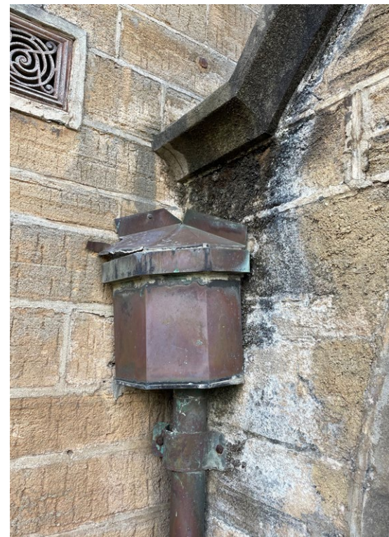
Salt deposition on limestone from gutter and downpipe overflow.
