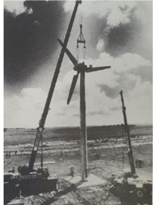
1987, Demonstration Wind Turbine being erected, Source: Solutions (newsletter of the Victorian Solar Energy Council).
