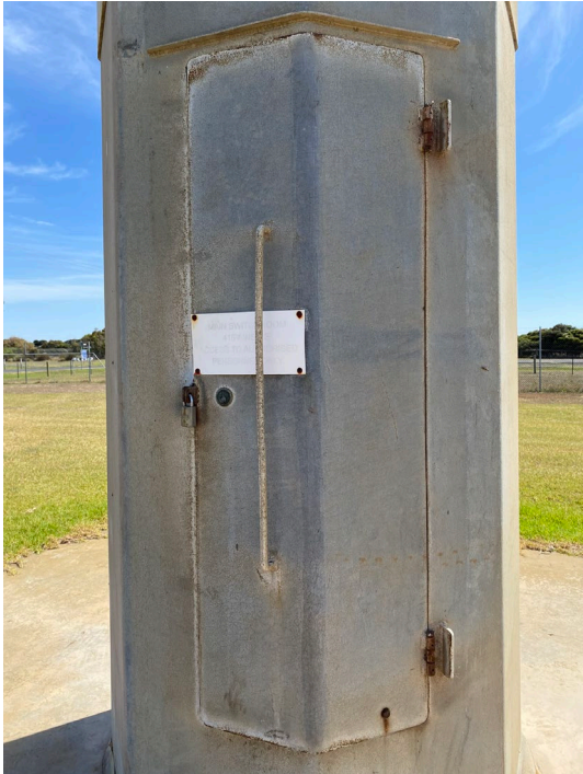
2025, the ground level access door of the wind turbine, Source: Heritage Victoria
