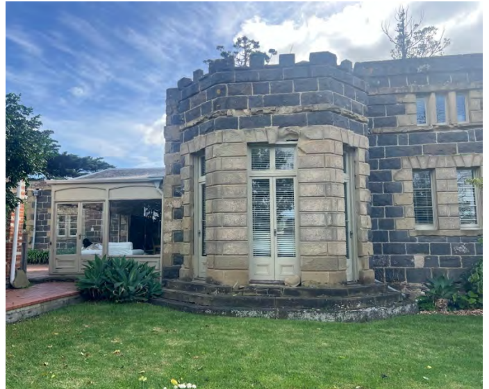
2026. Deterioration of sandstone around bay windows to the southern elevation. Source: HV.
