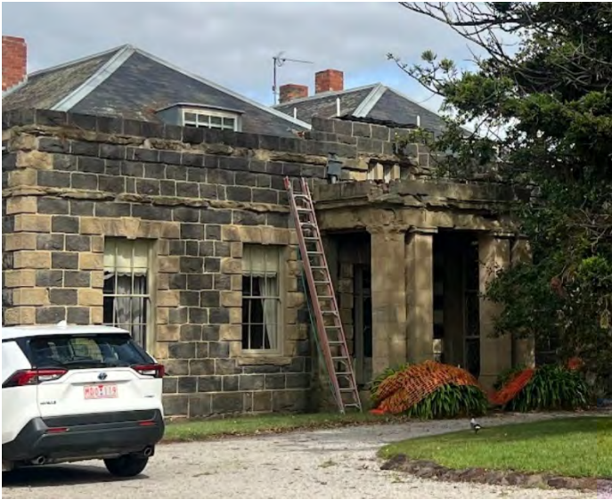
2026. Crumbling Barrabool sandstone to portico and mouldings. Source: HV.
