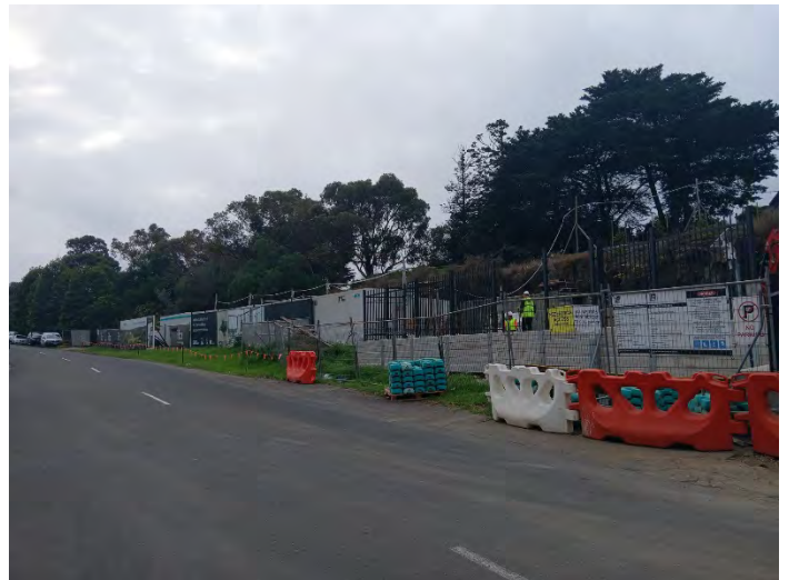
2025. Land beneath the steep embankment on Riversdale Road proposed for inclusion in the registered extent. Source: HV.
