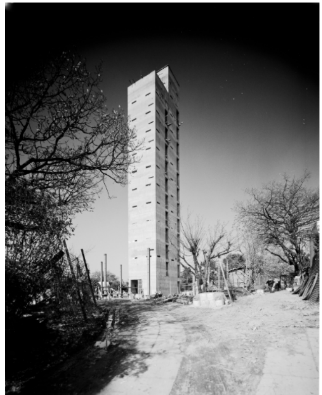
c.1962, construction underway with one of the service towers. Photographed by Mark Strizic. Source: State Library of Victoria.
