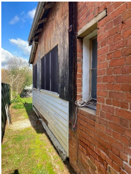
2026, Divide between original building and rear extension, Source: Heritage Victoria.
