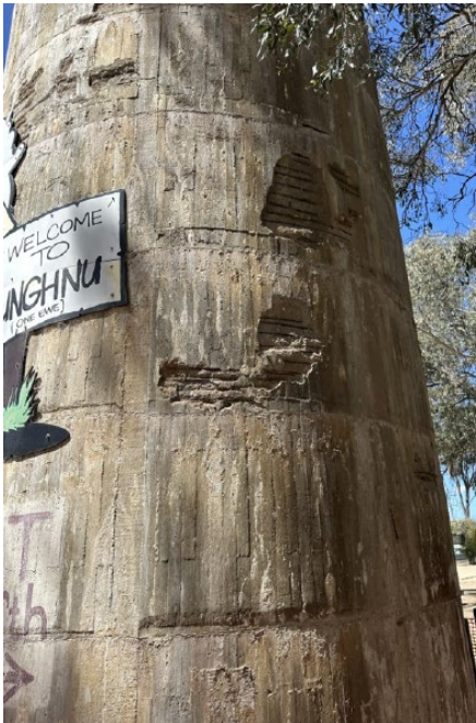
2024, Photograph of concrete loss. CAF Consulting Services, Structural Assessment Report, Wunghnu Water Tower, for Goulburn Valley Water, February 2024.
