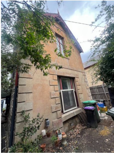
2026. 39 Nicholson Street façade with evidence of applied washes. Source: HV.
