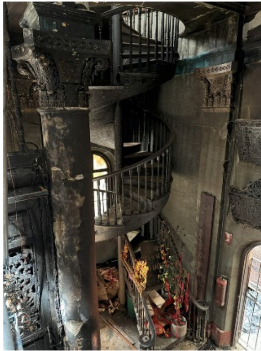
February 2024, Guan Di Hall, spiral staircase after the fire. Source: Sophie Couchman
