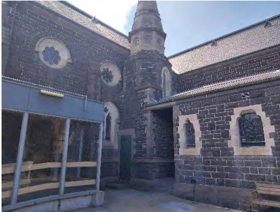
2024, View to the Convent Chapel from the aged care centre courtyard. Source: Heritage Victoria
