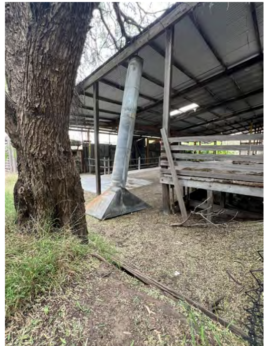
2024. Top Factory (6) back area of the building showing the relationship between platform and steam chambers.
