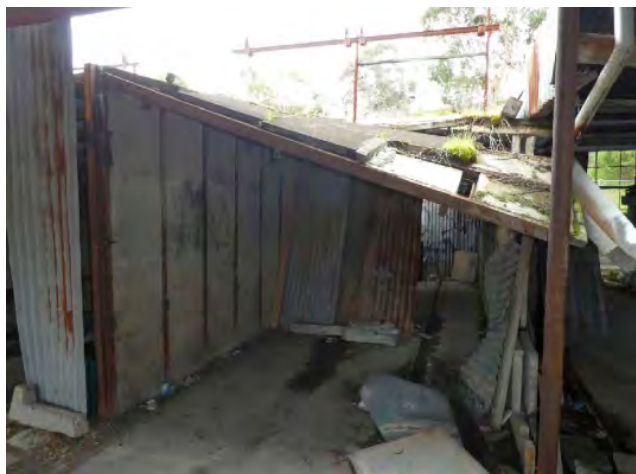
2022. Partial collapse of one concrete steam chamber to Top Factory. Source: FMG Engineering Investigation Report for Pipemakers Park.
