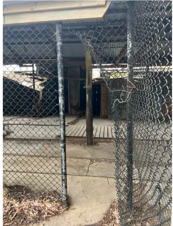
2024. Top Factory interior (6). To the left is a concrete steam chamber that is collapsing. Tramways to the floor.
