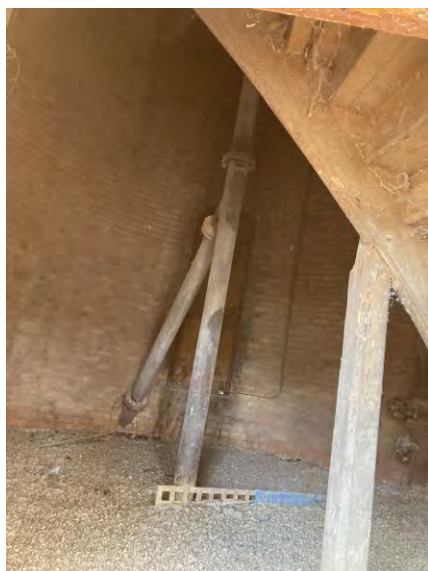
2023. Internal view of the tower shows the piping and staircase. The pigeon droppings are visible on the bottom.
