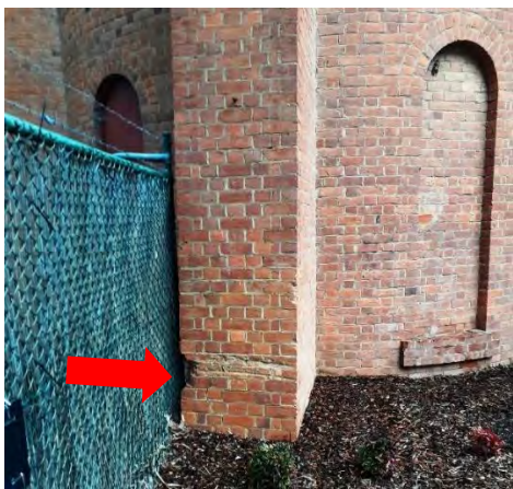
2023. Minor damage to the buttress is indicated by an arrow. Source: Nominator's collection
