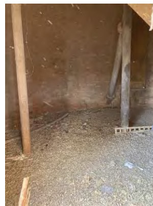
2023. Internal shot shows the extent of pigeon dropping.
