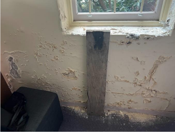
2024. Damp around window in northwestern ancillary room.
