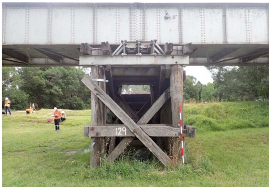
2017, Section of 1888 bridge showing timber piers and iron girder above. Source: AJM Joint Venture
