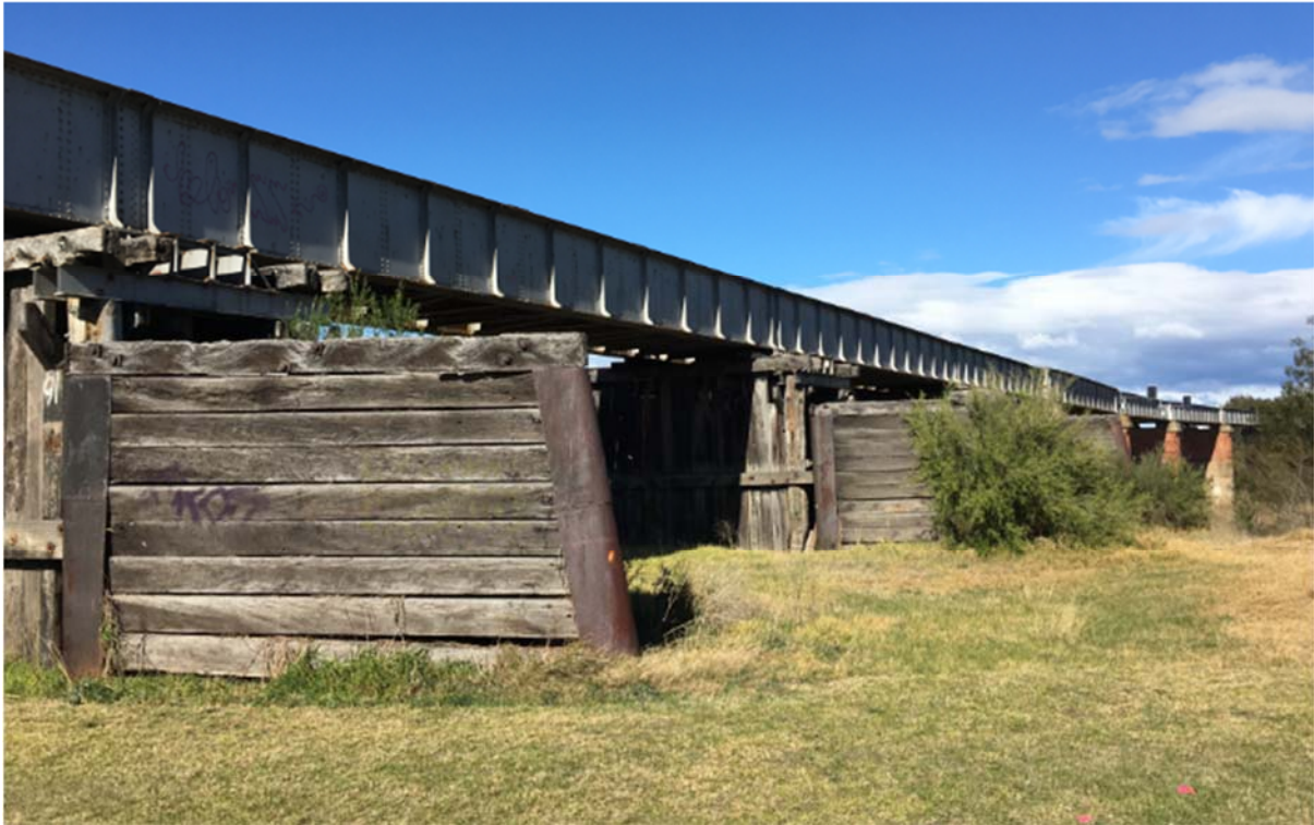
2018, Timber cutwaters and piers of the 1888 section. The 1896 section is at the right of the image.
