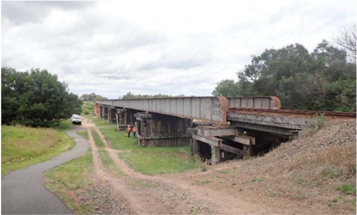
2017, Northern approach, 1888 section (Stratford side of the Avon River) showing timber piers with protective planking.
