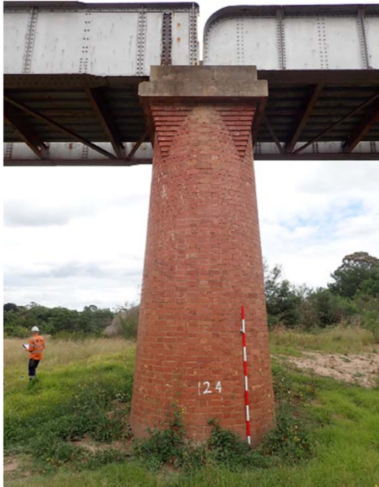
2017, Masonry pier supported 1888 girder (at left) and 1896 girder (at right). Source: AJM Joint Venture
