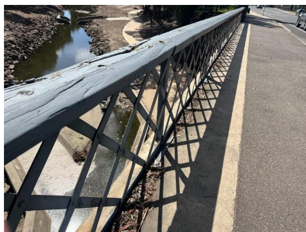
2024. Lattice balustrade, which was relocated to the northern (upstream) edge of the bridge during the bridge extension in 2004.
