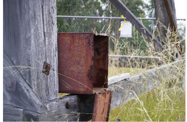
2025, the base of Mount Little Dick Fire Tower. The metal cabinet likely housed communications equipment. Source: Andrew Martin, DEECA
