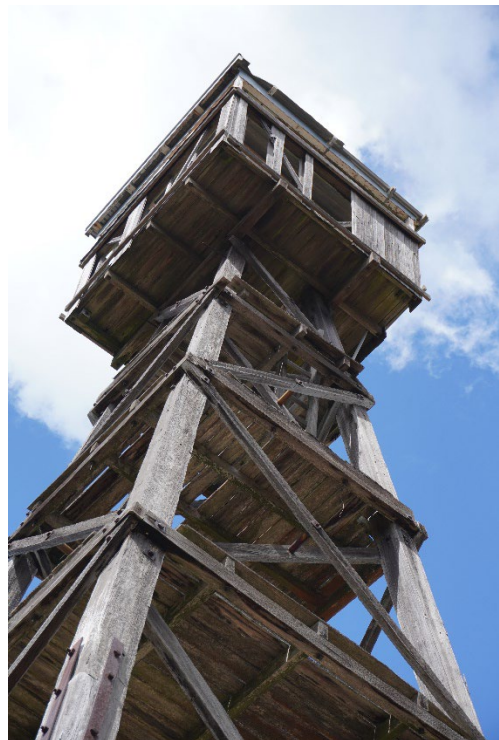
2025, the Mount Little Dick Fire Tower, detail of cabin. Source: Andrew Martin, DEECA
