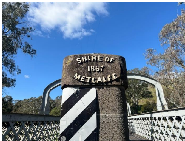
2024. Bridge pillar on the Metcalfe Shire side, bearing incorrect year of opening.
